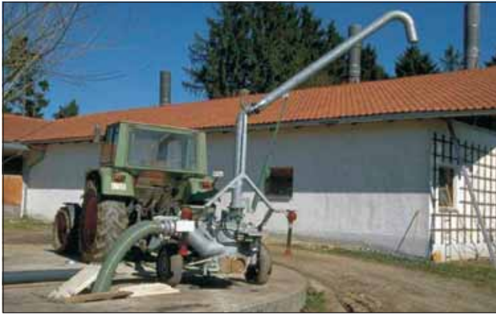
Pumpstation am Traktor
